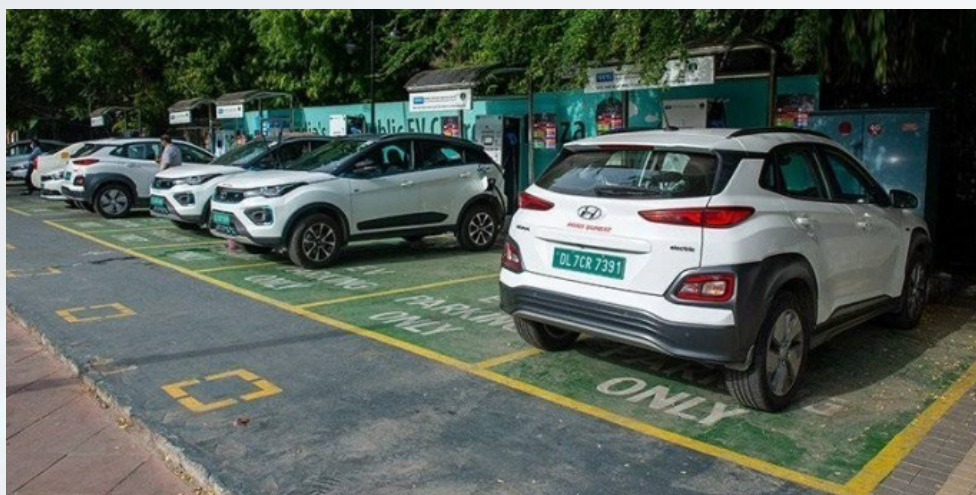
Charging stations set up by myGate for a residential complex
